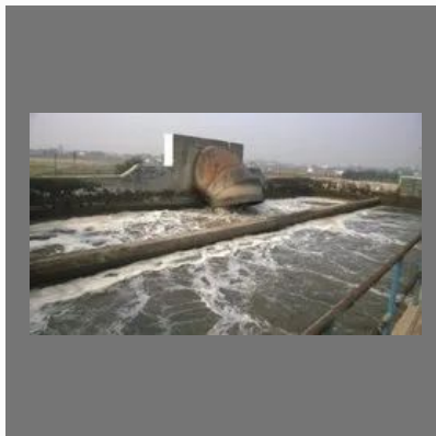
Effluent Treatment Plant System
