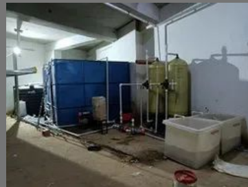
Commercial Sewage Treatment Plant
