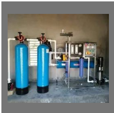
UV RO Plant
