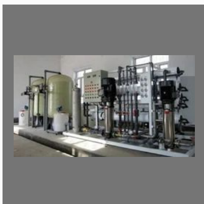
Water Treatment Systems
