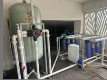
Water Filtration Plant
