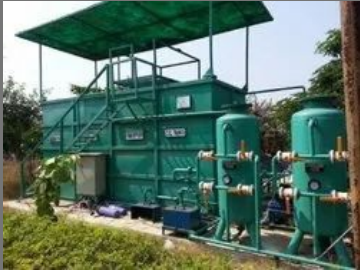
Effluent Treatment System
