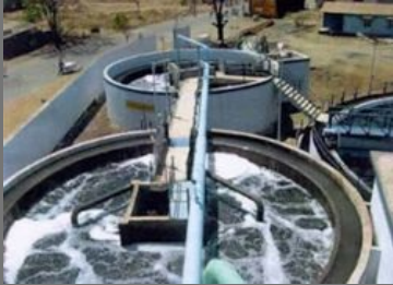
Effluent Treatment Plant
