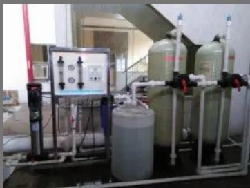
DM RO Plant
