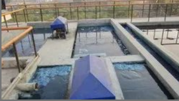
Industrial Water Treatment Plant
