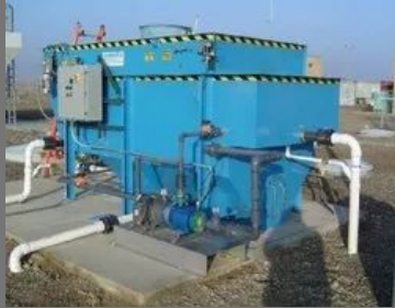
Compact Sewage Treatment Plant
