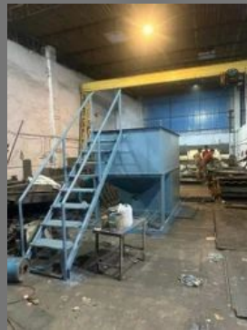
Effluent Treatment Plant
