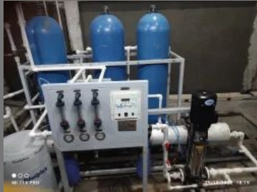
Ro Plant Filter
